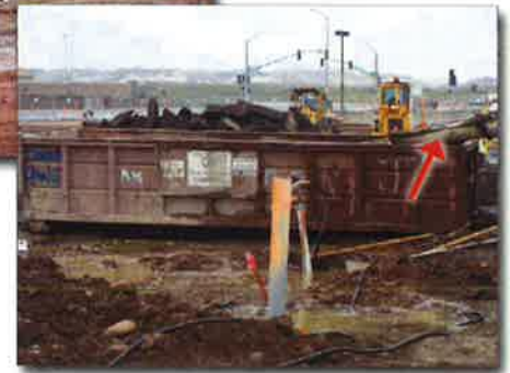
Figure 2. Chute washwater leaking from a roll-off bin being used as a washout container
