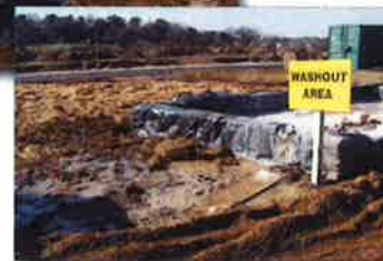
Figure 10. Leaking washout pit that has not been well maintained
