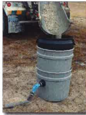
Figure 3. Concrete washout filter
