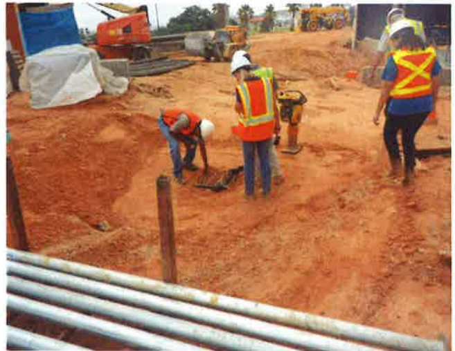
Construction staff inspecting a storm drain with inlet protection in an active construction area.
