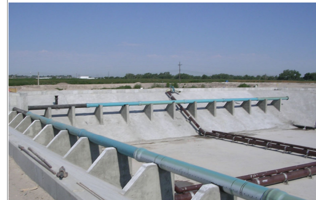
Waste Water Treatment Plant Aeration Basin
