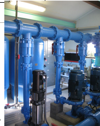
Monument Heights Water System Booster Station
