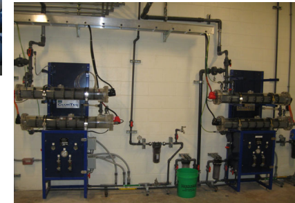
Drinking Water System Chlorine Generators
