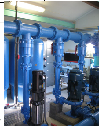
Monument Heights Water System Booster Station
