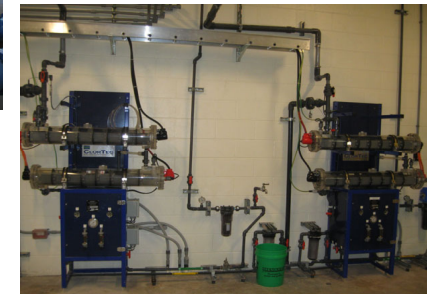
Drinking Water System Chlorine Generators
