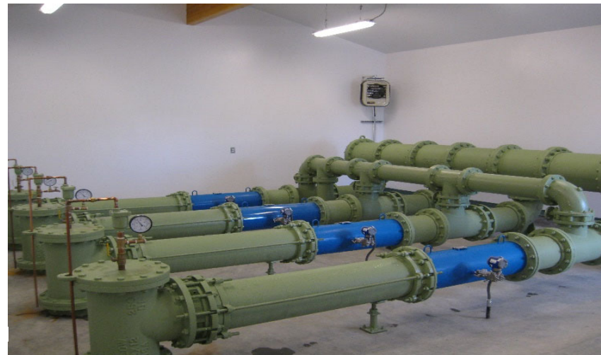
Gueck Meter Station
